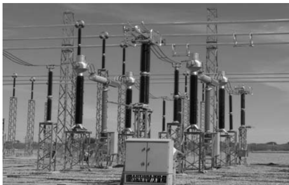
Figure 2. A Modern HVDC substation utilising the IEC 61850 Standard
